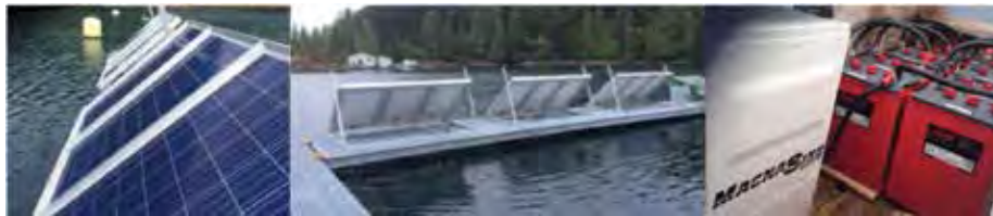
Installed renewable energy system components at Kyuquot SEAFoods Ltd. site: modular solar panels on dock (left and middle) with battery storage and power electronics in locker (right). Photo: Stephen Cross (UVic)
